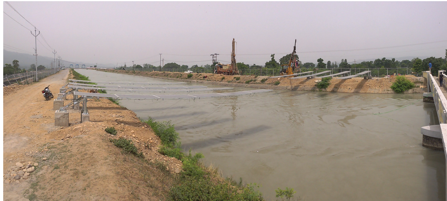
P.V. Over Canal Project in Gujarat, India https://www.apsunsys.com/en/references/
