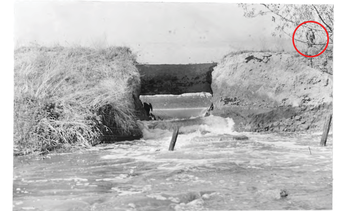
(1) Canal waters running out of break in Klamath "A" or Main Canal. View from property of Edward O. Thill (see item #1 of Appraisal of Damages), looking in a northeasterly direction. Dark area in center of photograph shows portion of gunite lining which held.
