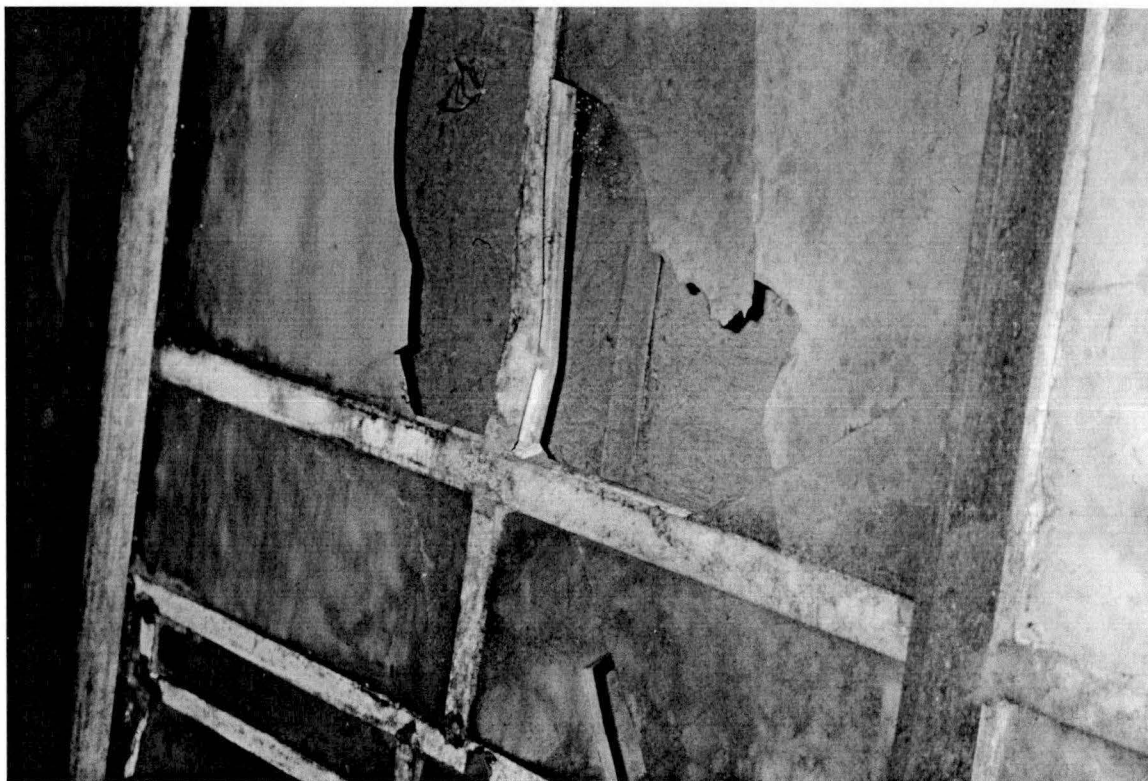
Figure 42. These Povey windows were removed from Johnson Hall at the University of Oregon and stored, unboxed, in a leaky warehouse for many years.
