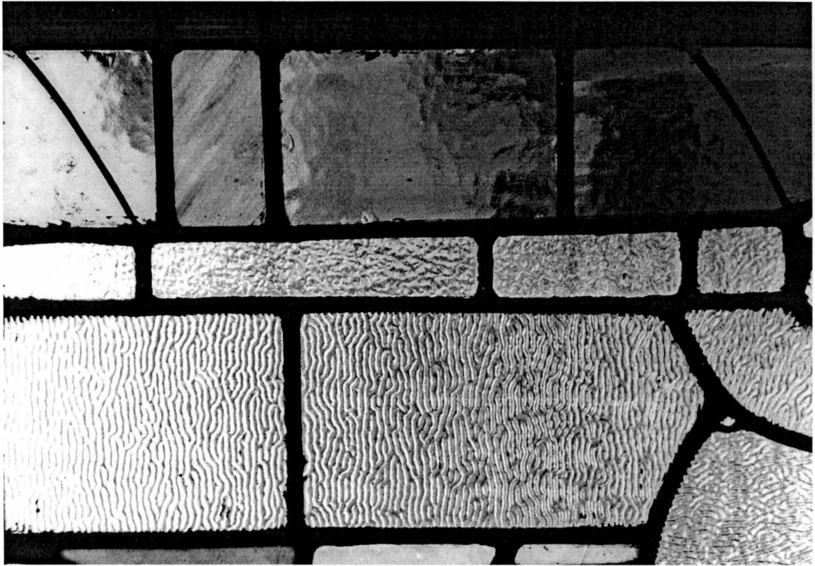
Figure 66. Old repairs are visible along the top of this window.
