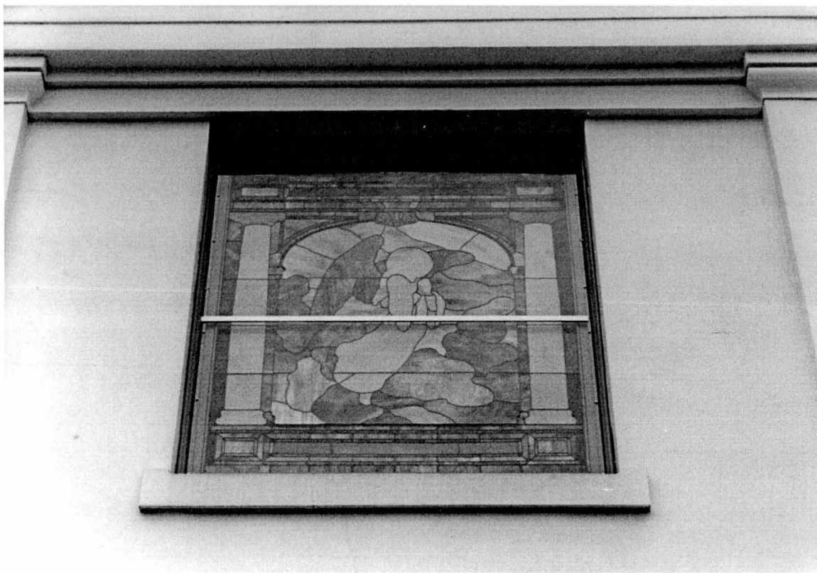
Figure 64. Protective glazing covers the sanctuary windows on the exterior.
