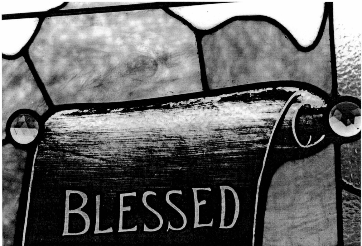
Figure 58. Damaged paint is visible along the top of this scroll in one of the 1897 windows.
