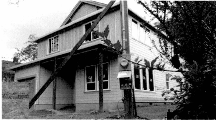
Figure 8. A new single-family home construction located at 8515 SE 21st Ave., Portland Oregon. photo taken by author, April 2016.
