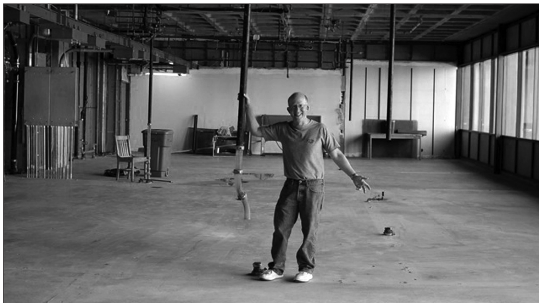
Department Head Mike Haley gestures in the site of offices and classrooms that were demolished to make way for the new general chemistry teaching labs.
