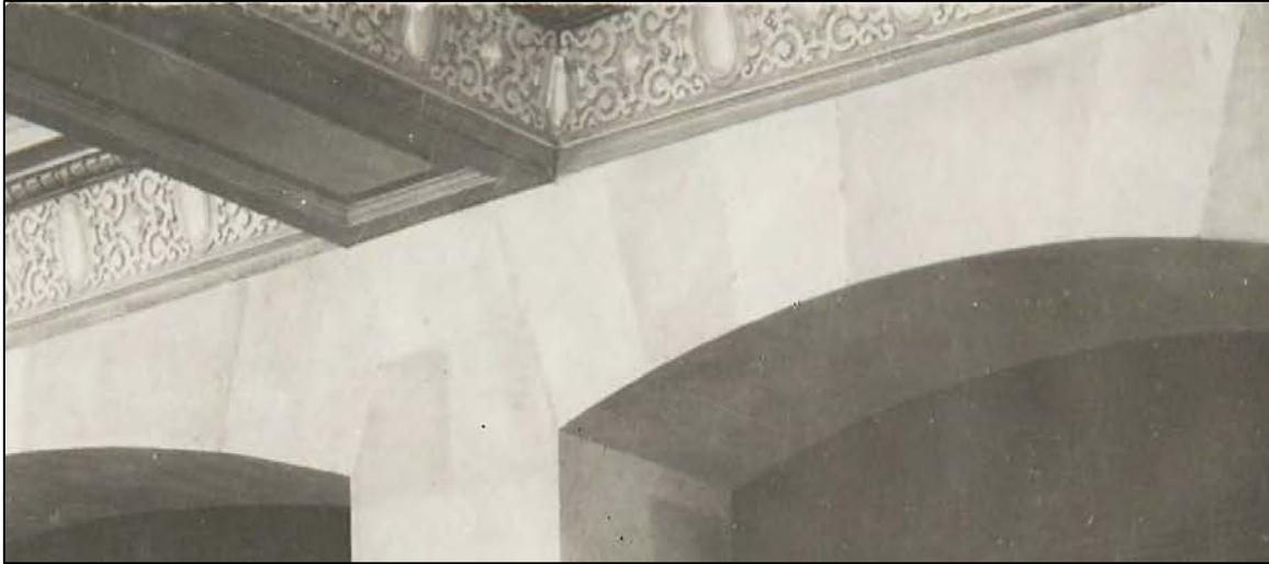
Figure 6. Historic view of Alumni Lounge looking west to the stairs, detail of cornices. Note the variation in value on the cornice, indicating different paint colors than the white used today. Most likely pre-1934. Image courtesy of University of Oregon Special Collections.
