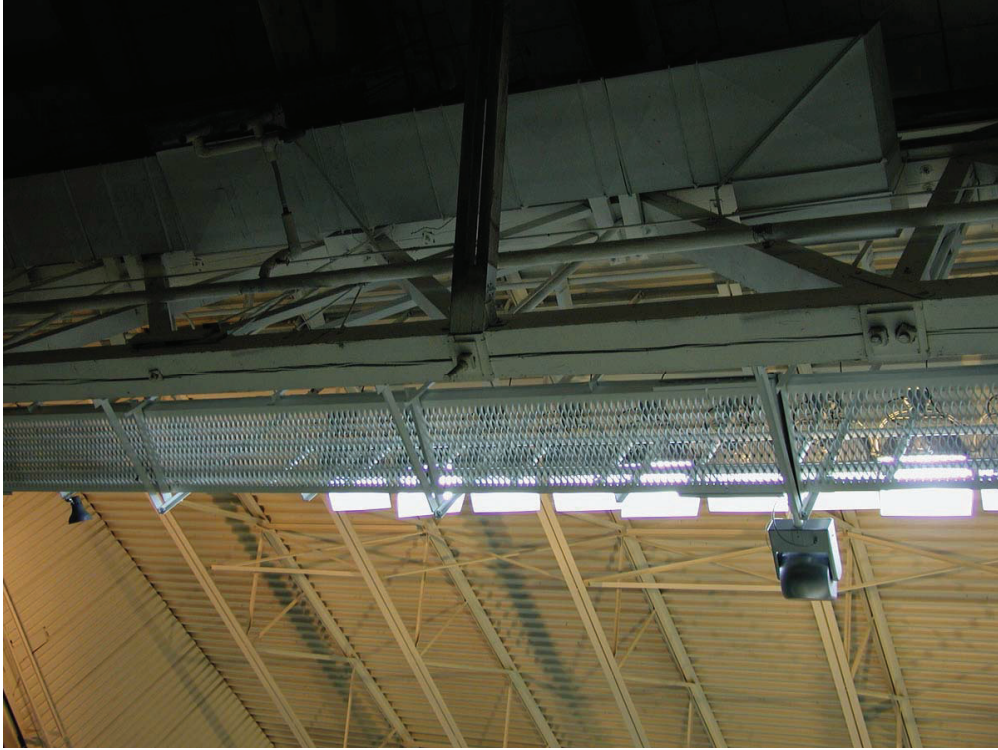
Photo 7 – Split in Bottom Chord
