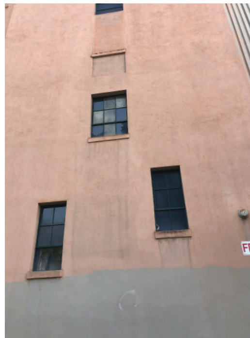
Window glass coverings/aging on glazing; biologic staining on stucco; finish/color differences
