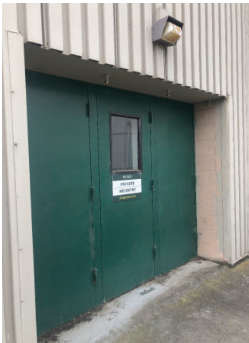
Incompatible light fixture; corrugate metal material
