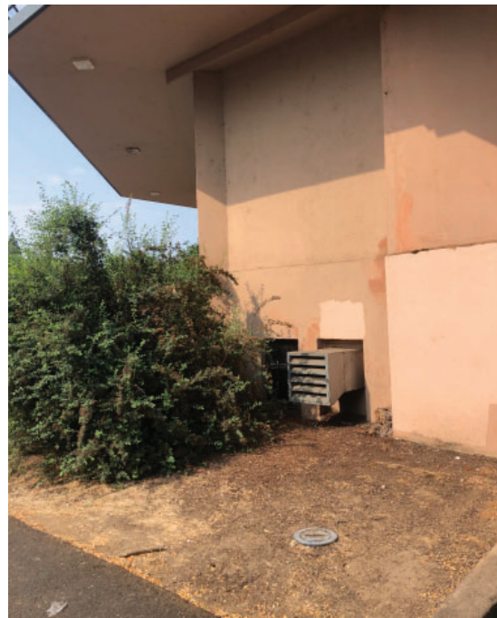
Exterior utilities and light fixtures
