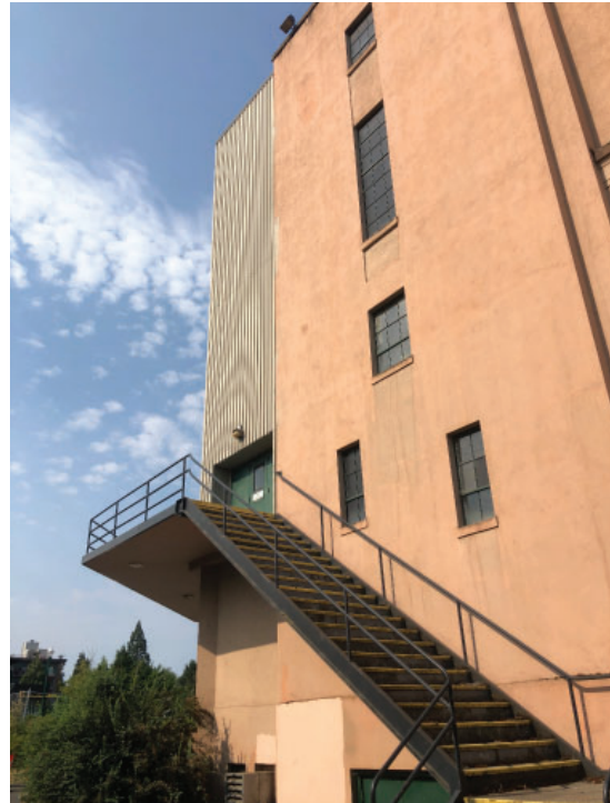
Stairwell leading up to corner stair tower and concrete landing additions at all four corners of building; corrugated metal material
