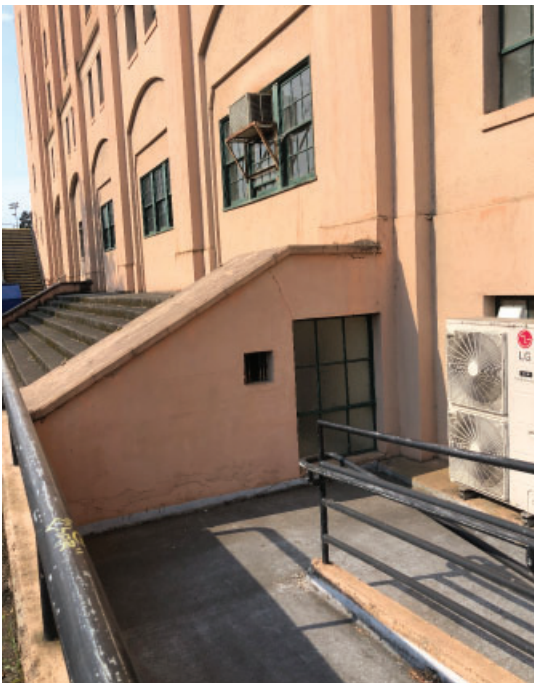
Exterior casement AC units
