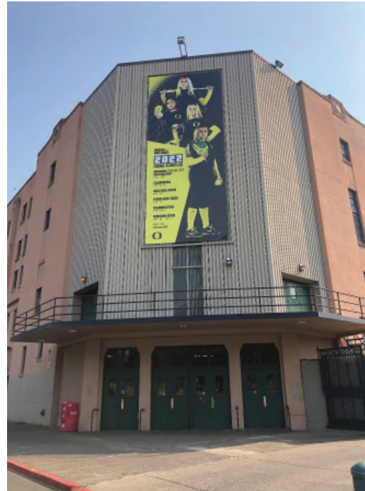
Corner stair tower and concrete landing additions at all four corners of building; corrugated metal material
