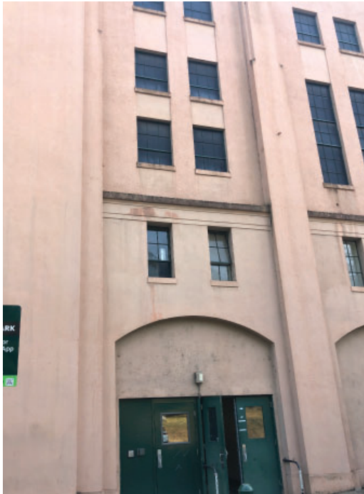
Incompatible light fixture; stucco repairs; biologic staining on stucco
