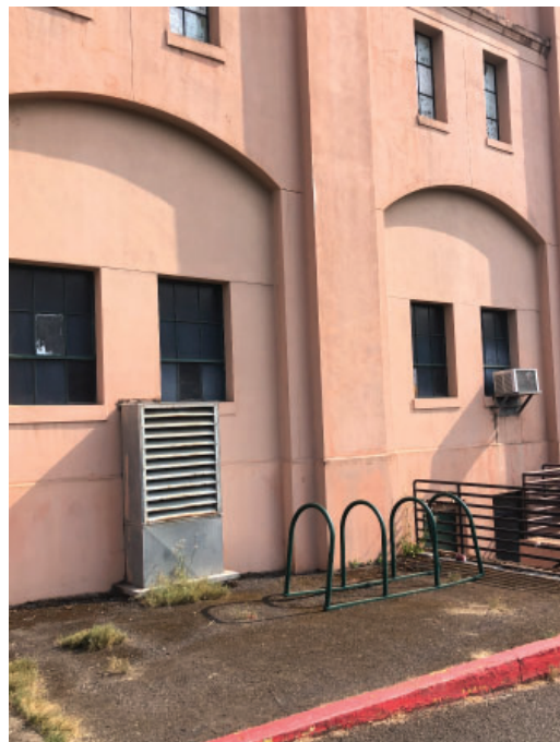
Exterior AC units and utilities
