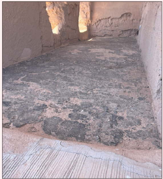
Crumbling asphalt on the interior of the Great House.
