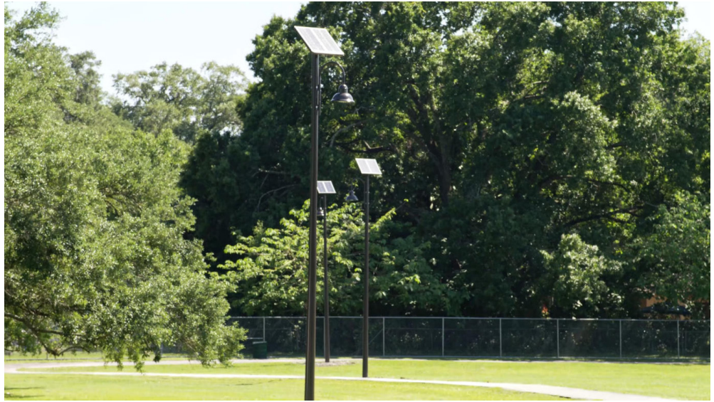
FIG. 9 Woodland Terrace Park solar powered lighting
