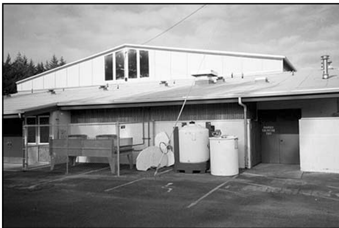
Equipment stored adjacent to this low roof provides easy roof access, inviting trouble.
