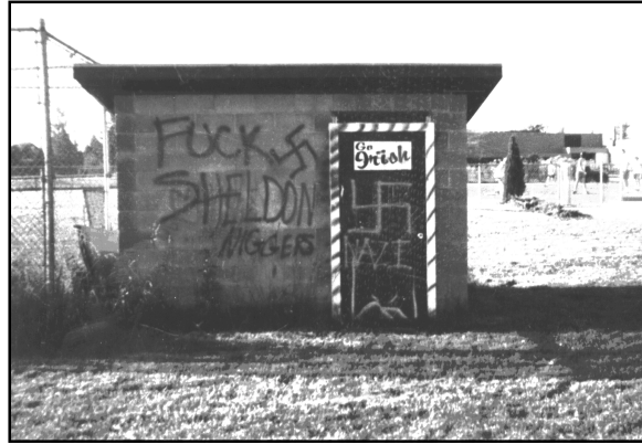
Extensive hate graffiti undermines school climate and territoriality.
