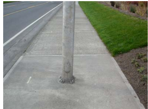
Pathway obstruction on Meadows Rd.
