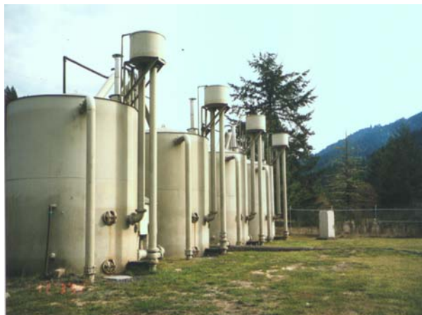
Filters at lower site
