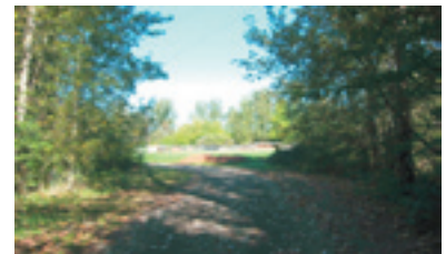
The gravel road that separates the east and west pond. The culvert is under the road.
