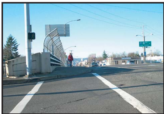
C View to the west of sidewalk on the south side of Sandy Boulevard.
