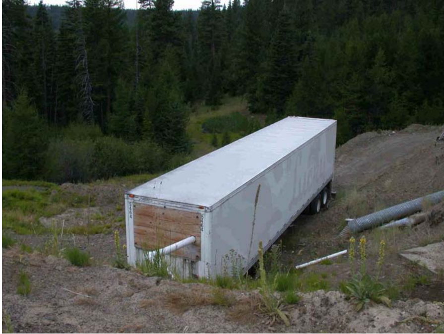
Photo 7. Water treatment facility (Photo by D. Boles)
