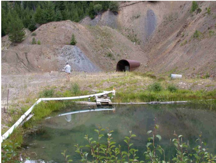
Photo 4. First treatment pond below the 600 Level Portal (Photo by D. Boles)
