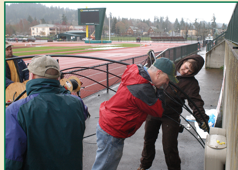
Don Williams (red jacket) works with an IES Security employee (right) to feed cable into the conduit in the west Hayward Field grandstand as part of the larger wiring upgrade project. Information Services installed several kinds of cable for a variety of purposes. The new scoreboard alone (shown in the background) required fiber optic, cable TV, phone wire, and custom cabling.
