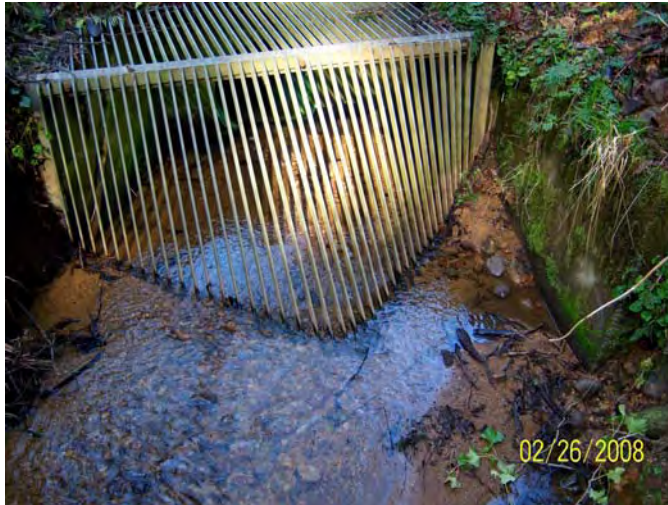
Figure 5. Stormwater drains – Astoria, Oregon
