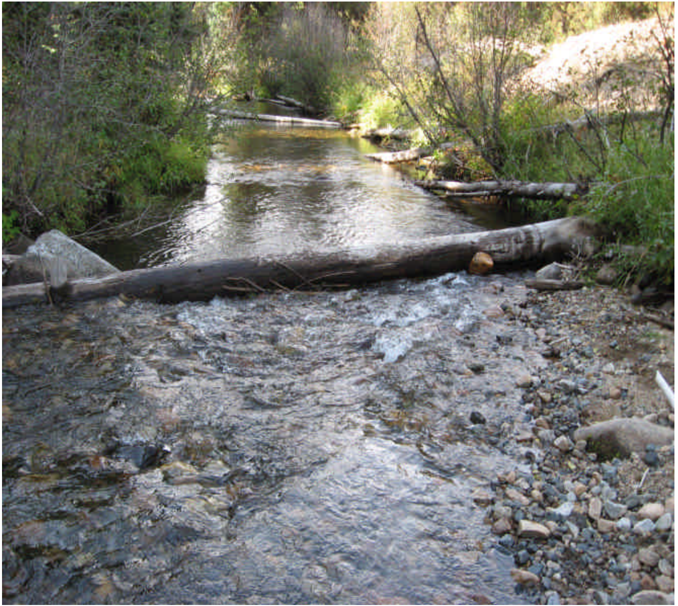
Failed structure. The middle of the log will be removed. One root wad with log attached and 3 – 50' logs will be added to structure to maintain a pool, provide cover and narrow the channel.
