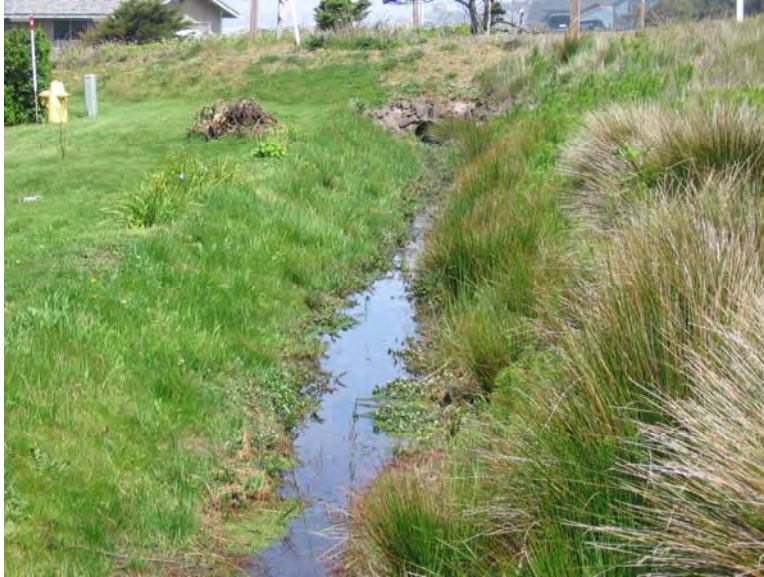
Figure 3.1.7-Mainline Culvert at corner of Yachats Ocean Road and HWY 101 Note the ditch free of major obstructions
