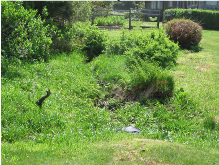
Figure 3.1.1-Mainline Culvert at Yachats Ocean Road Note the restricted ditch line upstream of the culvert inlet
