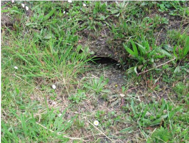
Figure 3.1.4-Mainline Culvert along HWY 101 near Cape Ranch Road Note the obstructed culvert inlet
