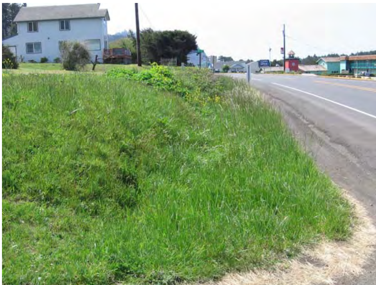
Figure 3.1.2-Mainline Culvert Located at 232 Highway 101 Note the obstructed culvert inlet
