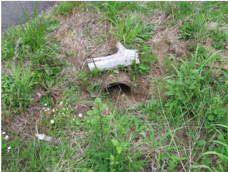
Figure 3.1.2-South Side Cape Ranch Road Note the obstructed culvert inlet
