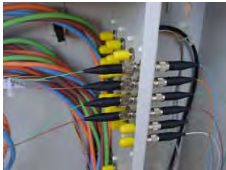
Fiber Optic Cable Terminations
