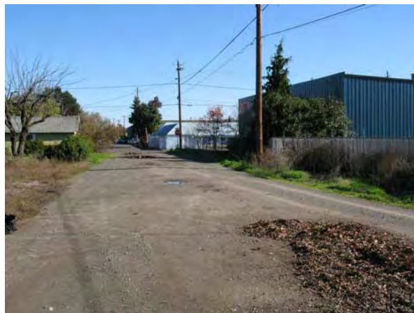
Typical unimproved street in Gateway Area
