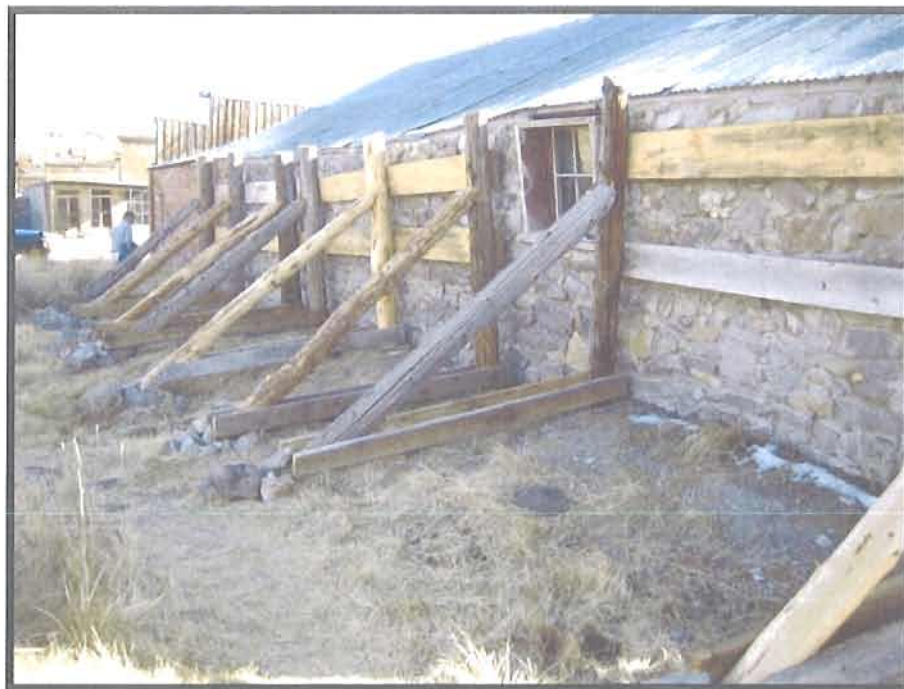
Figure 5.13. Pre-1962 stabilization efforts in Bodie, CA. Note the replacement of the historic stabilizing members, a practice consistent with retaining all features extant previous to State Park acquisition. Photograph by the author, 2008.
