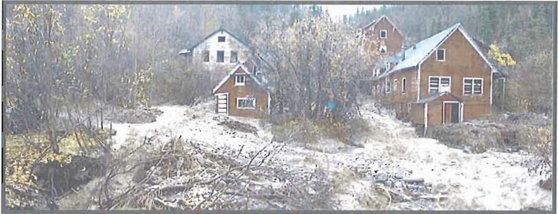
Figure 5.7. Buildings in the pathway of National Creek, Kennecott NHL. A severe flood in 2006 deposited massive amounts of gravel and damaged multiple buildings. Photograph courtesy of www.steliasguides.com .
